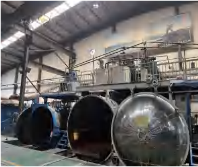
▲ 真空浇筑罐 Epoxy Resin Vacuum Casting Tank
