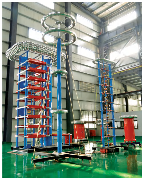
▲雷电冲击设备 Lightning Shock Equipment
